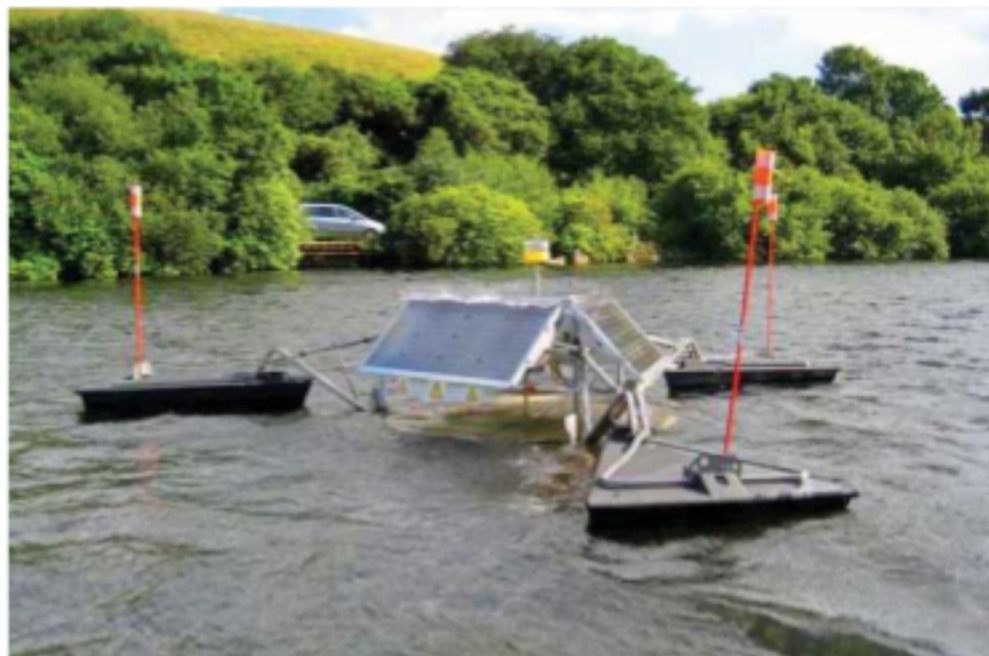
The solar-powered destratification system
